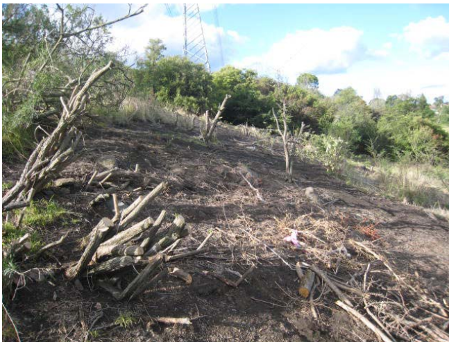
BELOW Removal of woody weeds in preparation for rabbit proof fencing and planting
